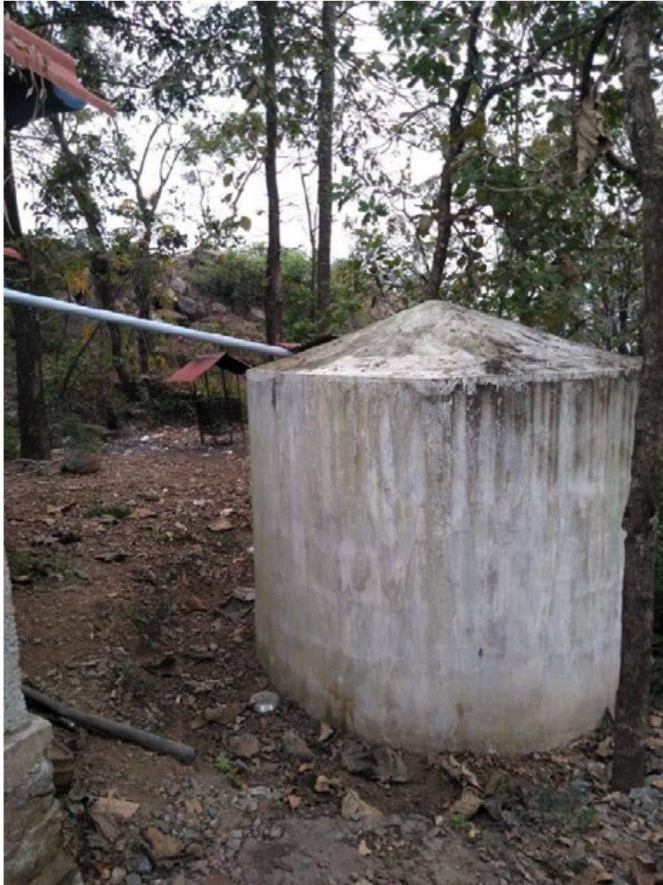
Photograph showing the rainwater harvesting tank
